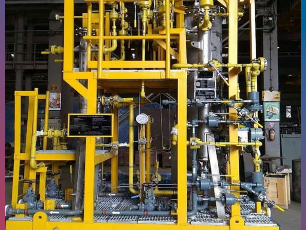
Instrument Utility Gas Drying Systems
